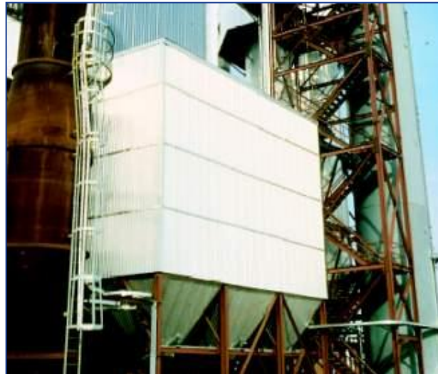
Coal-fired Industrial Boiler 110,000 ACFM
