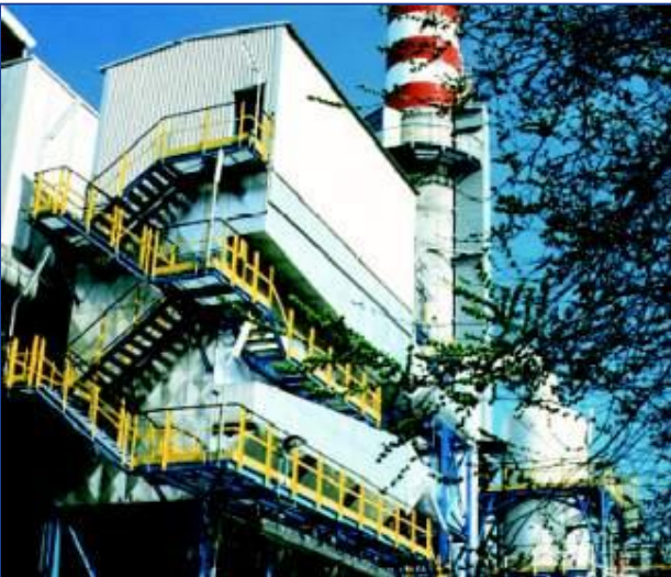
Municipal Solid Waste Incineration 16 MW – 65,000 ACFM
